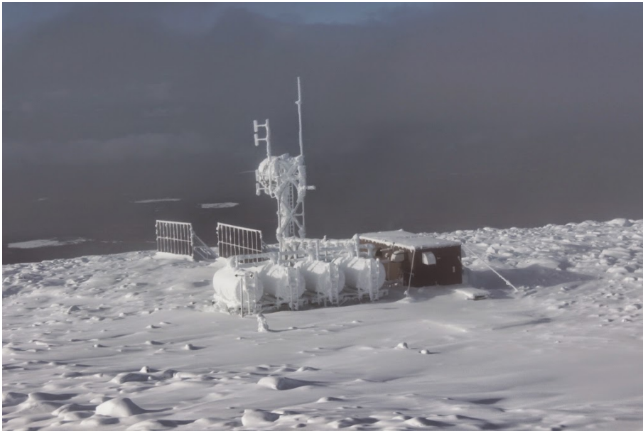
Left top: telecommunications repeater station at McEvoy Lake, Canada, in winter
