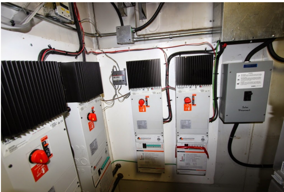
Left bottom: the installation's power bay with an array of Morningstar 600V charge controllers
