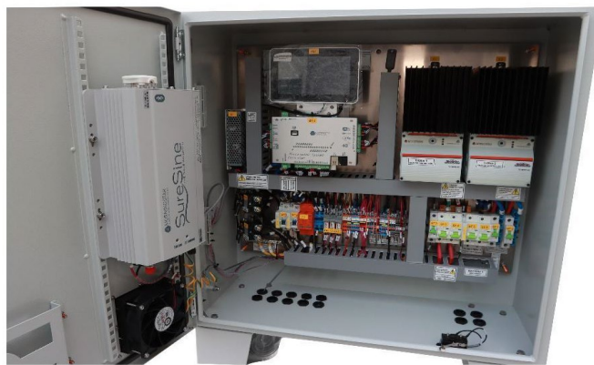
Morningstar SureSine inverter deployed in a remote telecommunications system
