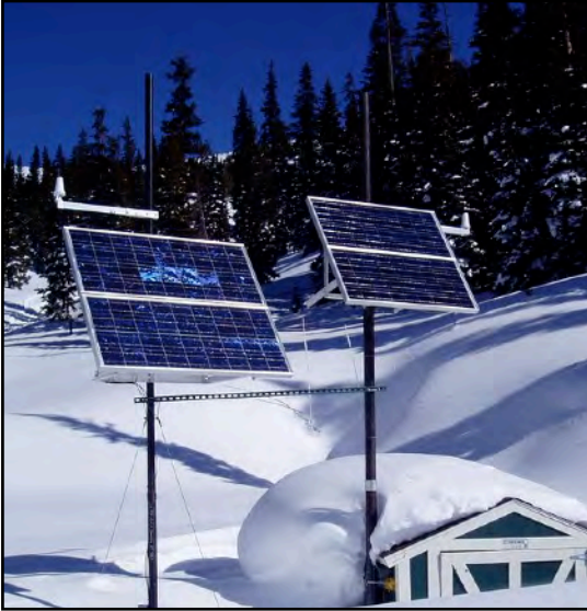
Photo courtesy of Nunatak Alternative Energy Solutions
